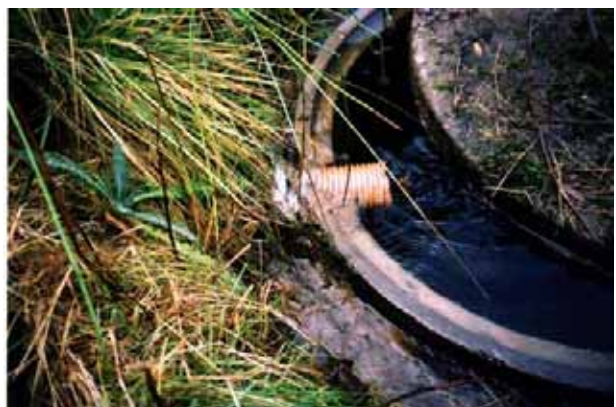
Water supplies set too low in the ground allow contaminated surface water to enter the collection chamber
